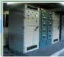
UNIVERSAL Floor Rubber Mat near Electrical Switchboard & Power House
