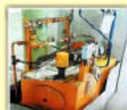
UNIVERSAL High Pressure Ball Valves in Hydraulic Unit
